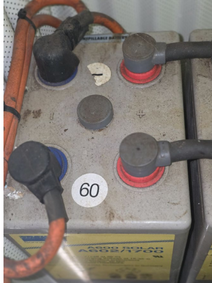
Figure 5. One of the 60 cells in the Mata Mata battery room (Sonnenschein A600 Solar A602/1700), sticker number 60. Photograph: Peter Botsman, October 2026.
