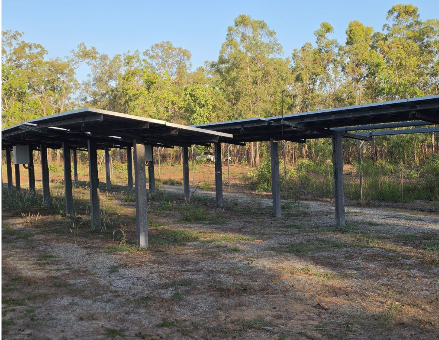
Figure 1. The Mata Mata solar array: rows of panels on raised steel frames in a fenced, cleared block at the edge of the bush. Photograph: Peter Botsman, October 2026.
