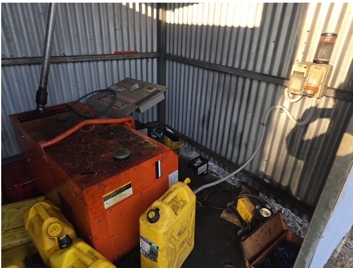
Figure 7. The backup diesel generator in its shed at Mata Mata, with jerry cans of fuel. During the October 2026 Bāpurru funeral it ran almost around the clock for at least seven days. Photograph: Peter Botsman, October 2026.
