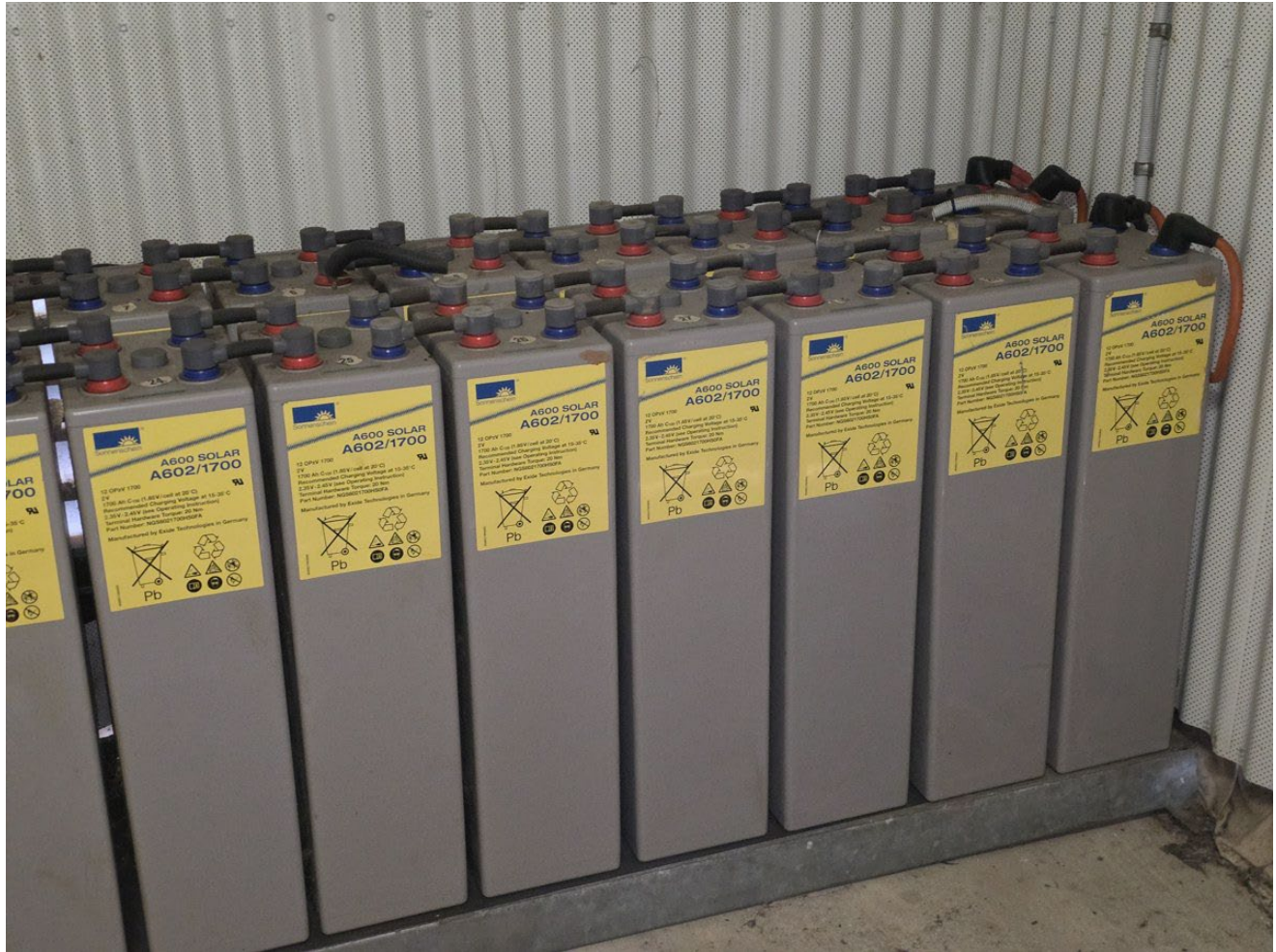
Figure 4. Part of the battery bank at Mata Mata: rows of Sonnenschein A600 Solar A602/1700 cells (12 OPzV 1700, 2 V, 1700 Ah at C100), made by Exide Technologies in Germany. Photograph: Peter Botsman, October 2026.
