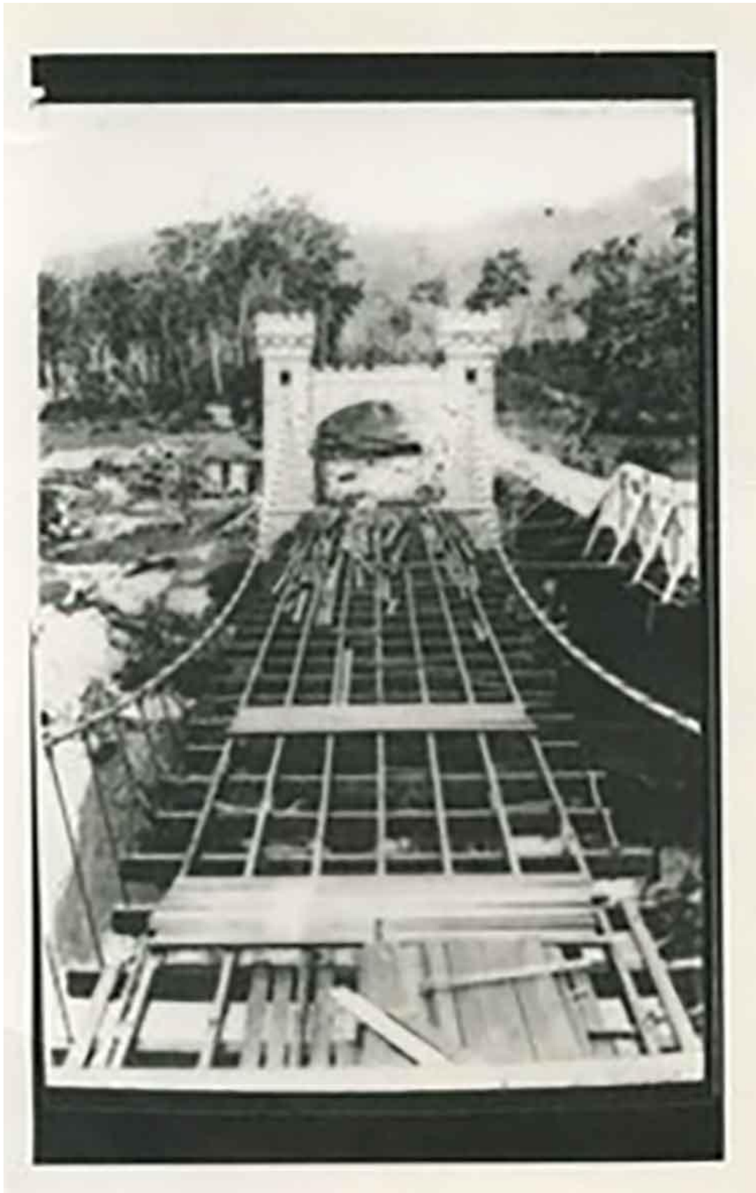
Image 17 A blurry but all important photograph of the original hard wood deck during construction with the original bridge still alongside c1897
